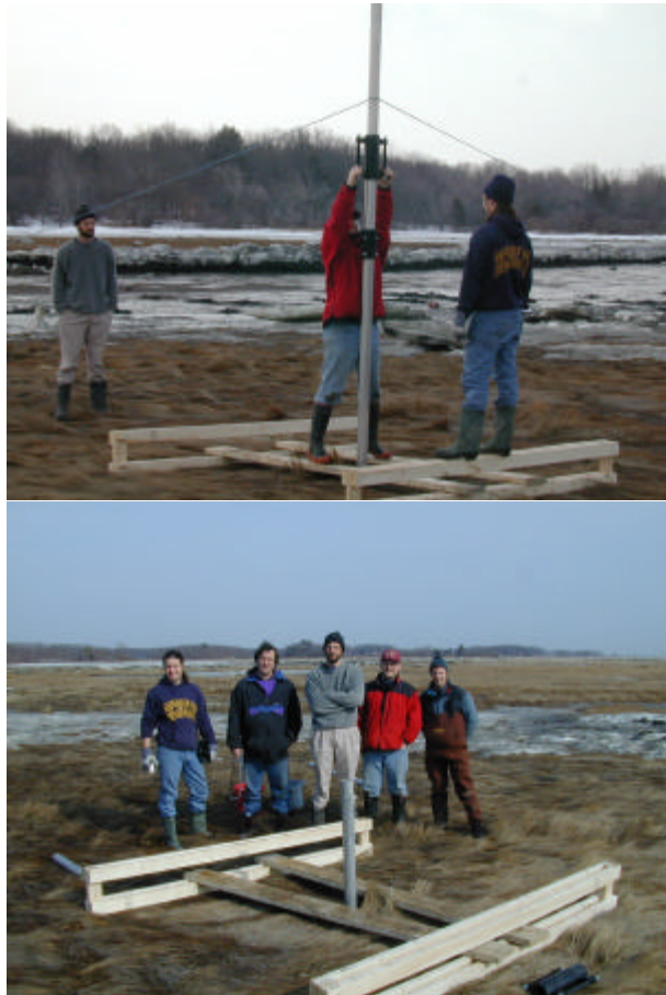
Figure 7. Installation of SET platforms in Plum Island marshes during winter so as to minimize disturbance to vegetation.
